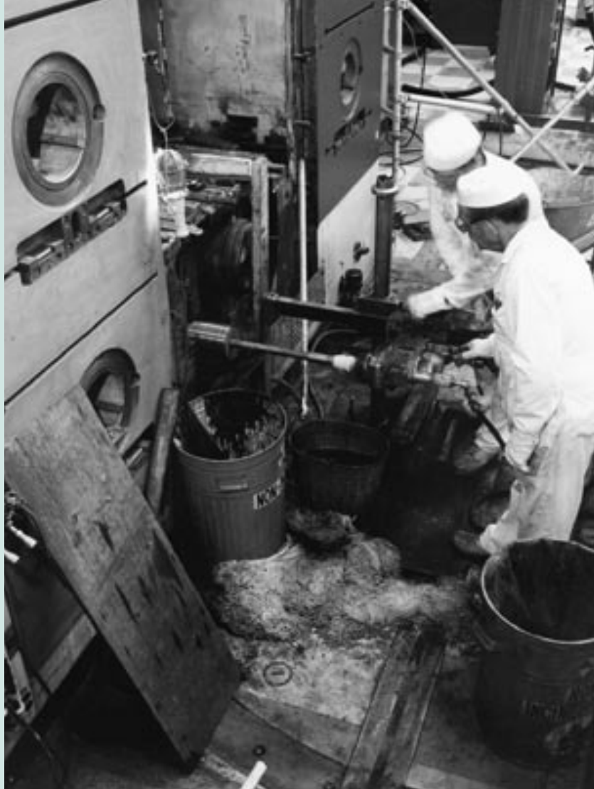
When the DUALSPEC instrument was installed in the early 1990s some modifications were made to the main concrete shielding of the NRU reactor.
